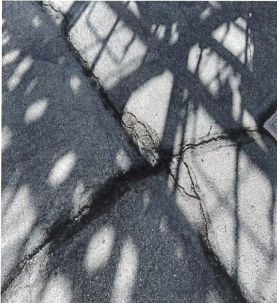
Sample of Cracked Asphalt at the Valley Station
