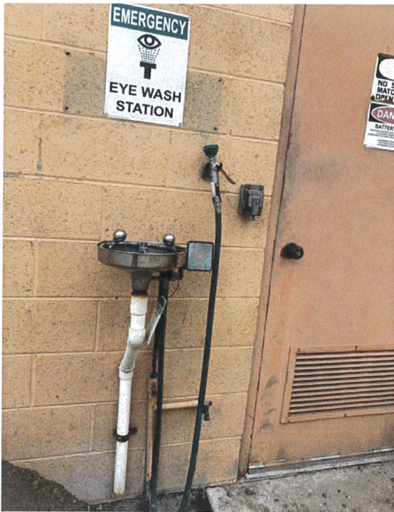
Old eye wash station at San Jose Station
