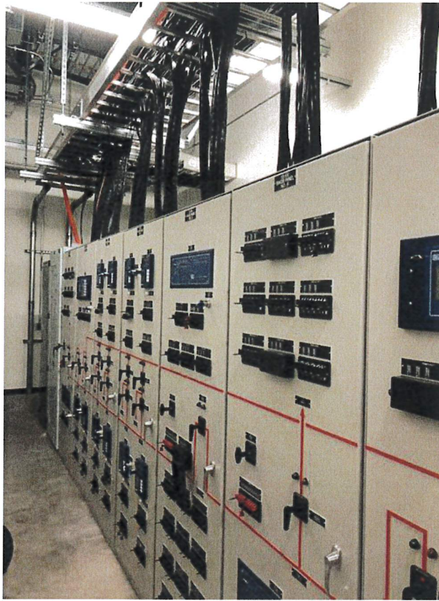
12kV Relay and Control Panels – Wiring Complete
