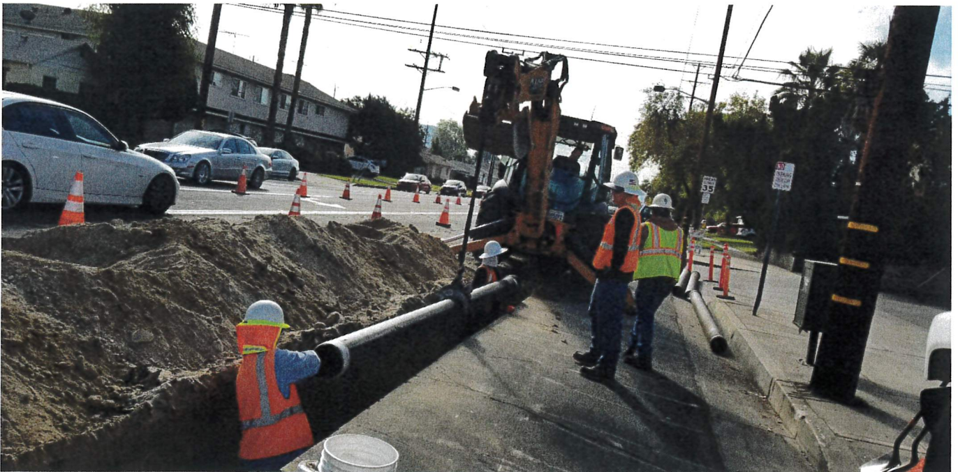
Installation of an 8-inch potable water main in Hollywood Way between Victory Blvd and Jeffries Avenue. Photos show the installation of an 18-foot-long section of 8-inch ductile iron pipe.
