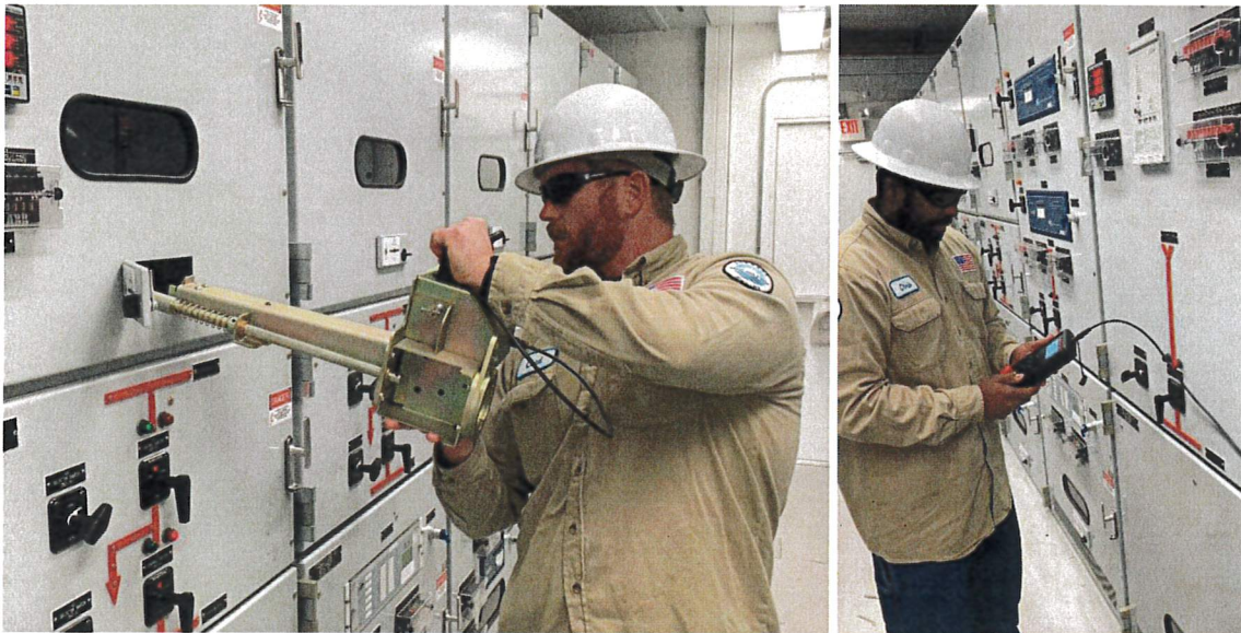
Racking motor and interface (Left), remote operating console (right)
