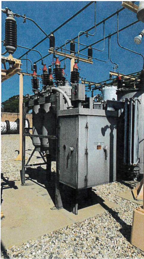
Old 34.5kV OCB
