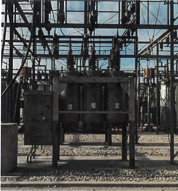
Original 34.5 kV Oil Circuit Breaker
