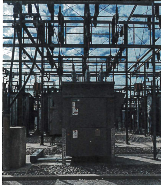
New 34.5 kV Vacuum Circuit Breaker
