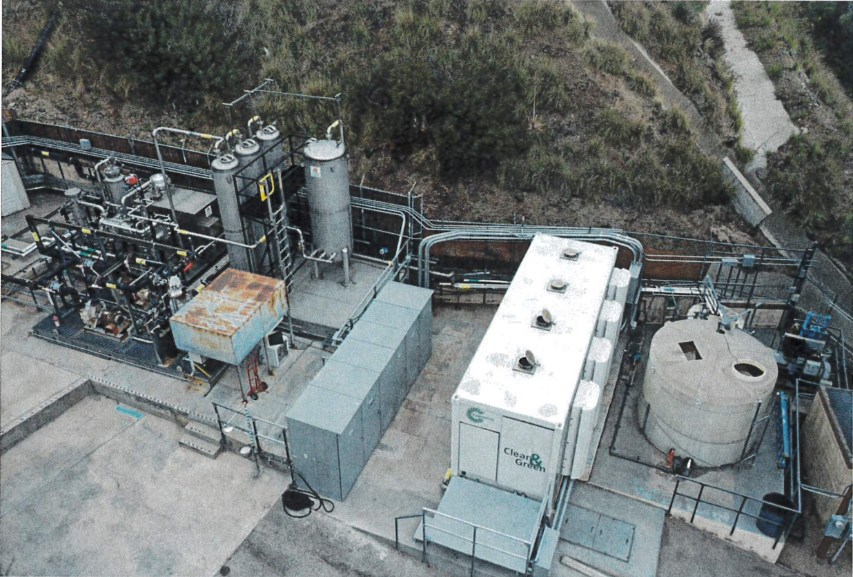
LFGTE Installed System
