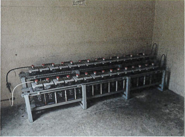
Battery Bank – Before Installation
