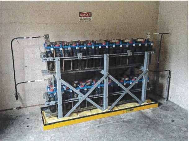
Battery Bank – After Installation
