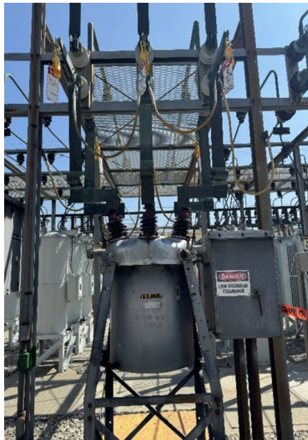
Old Oil Circuit Breaker
