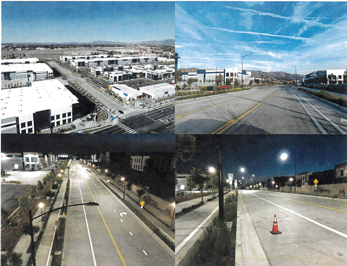
Above-left - Aerial photograph looking west from Hollywood Way/Tulare Above-right and bottom - Photograph of a new portion of Tulare at day and night with new BWP streetlighting
