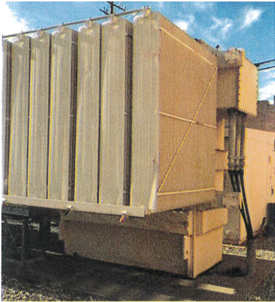
Old San Jose terminations
