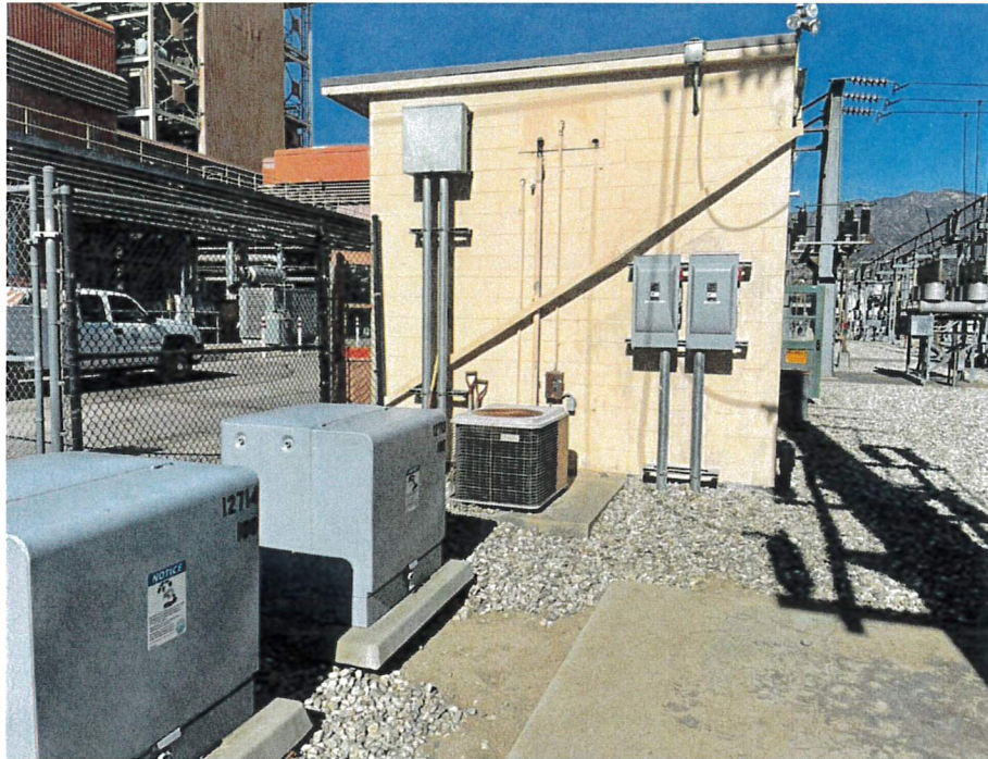
New Fused Disconnect Switch at Olive Sw. Substation
