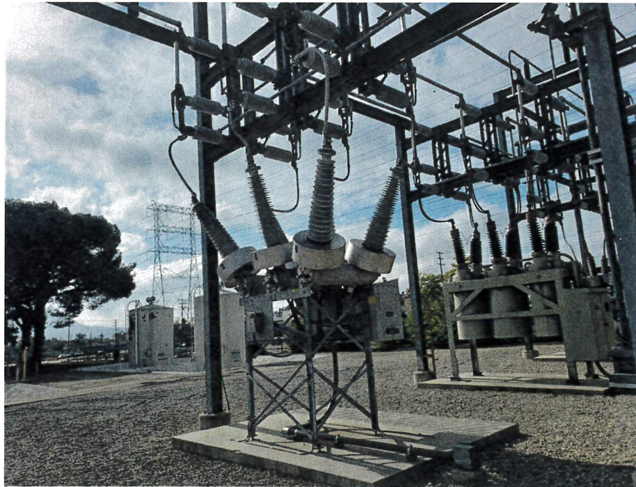
New Circuit Breaker Picture at RSE
