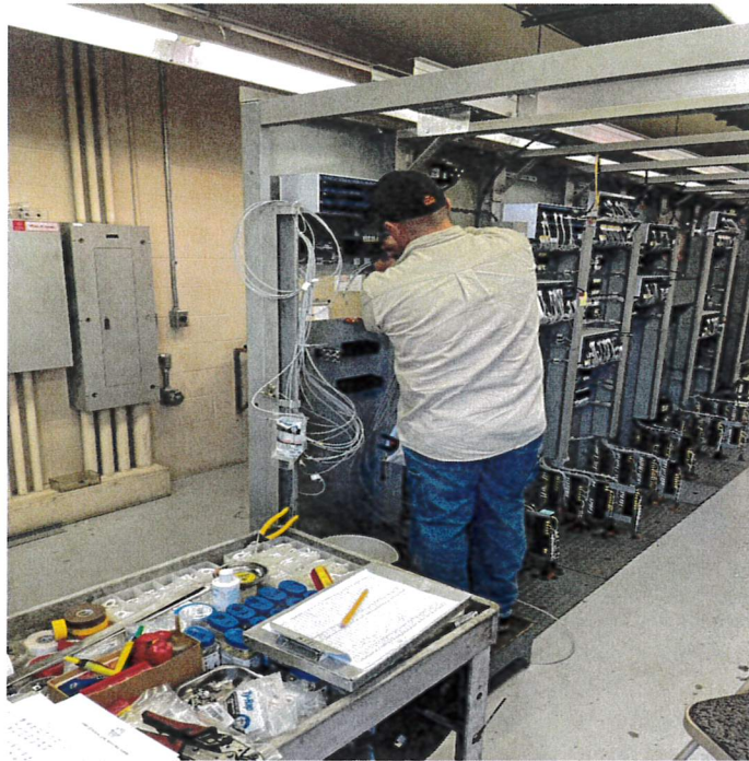
Panel Work at Lincoln for the Lincoln-Valley Relay Upgrade
