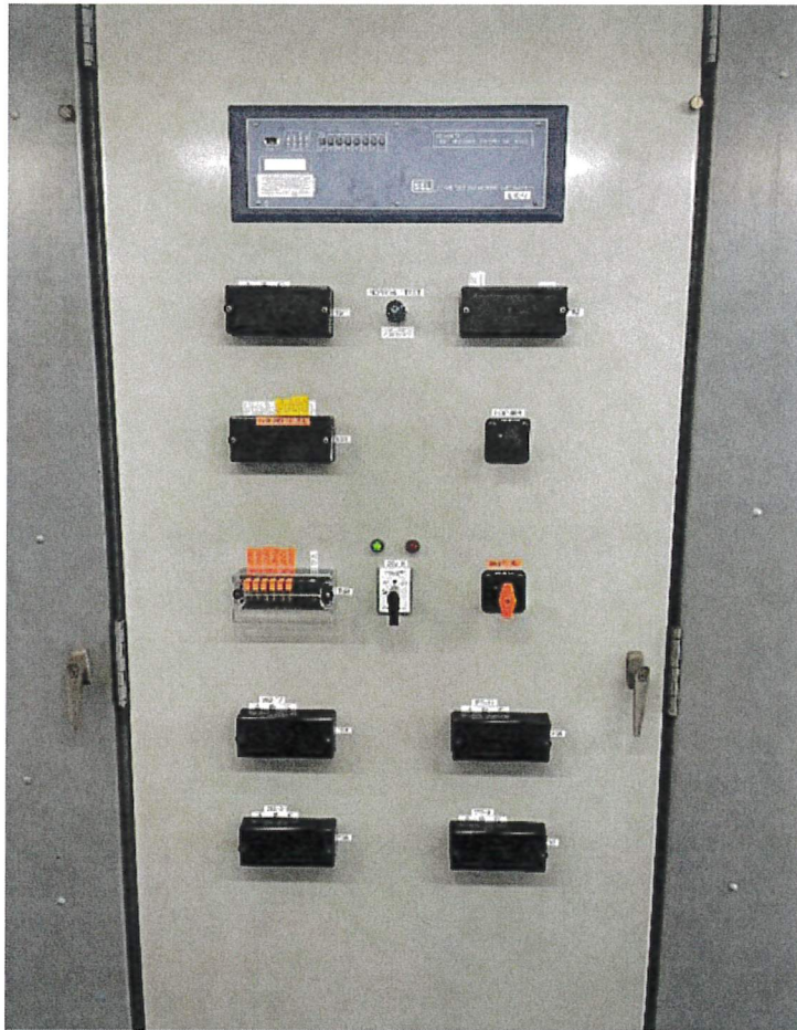
Breaker Fail Master Lockout at San Jose Substation
