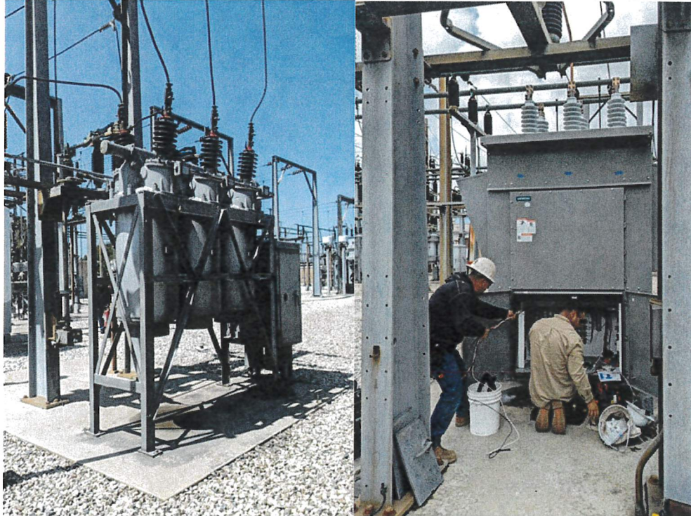
Old 34.5kV OCB Breaker at Valley Station
