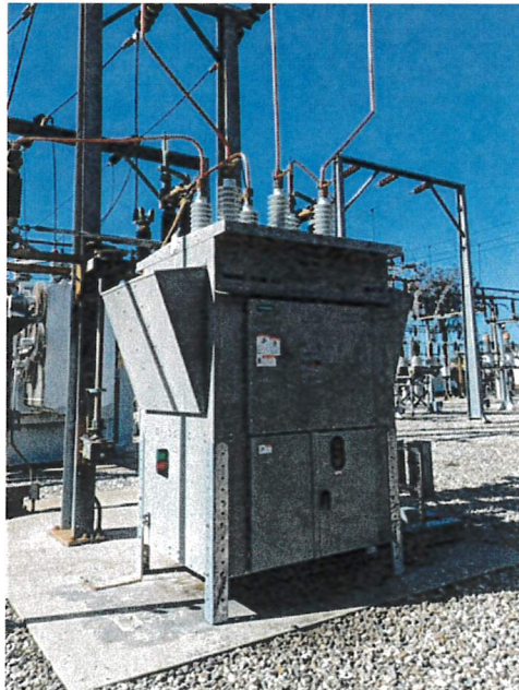
New 34.5kV VCB Breaker at Valley Station
