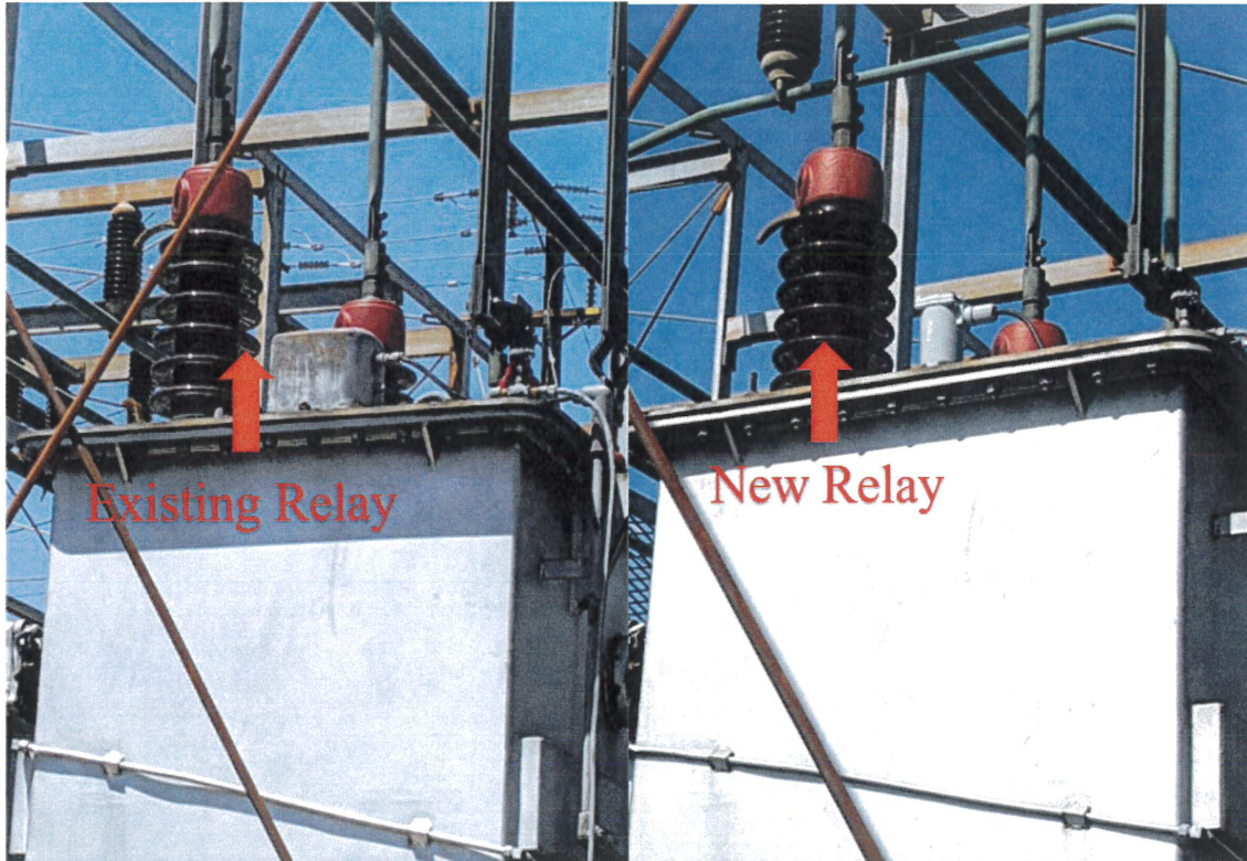
Old Sudden Pressure Relays at Winona A-3
