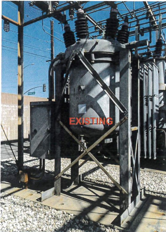
Original 34kV Oil Circuit Breaker at Winona Bk. A-1
