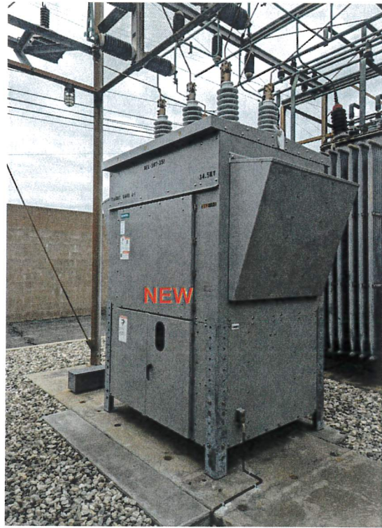
New 34kV Vacuum Circuit Breaker at Winona Bk. A-1
