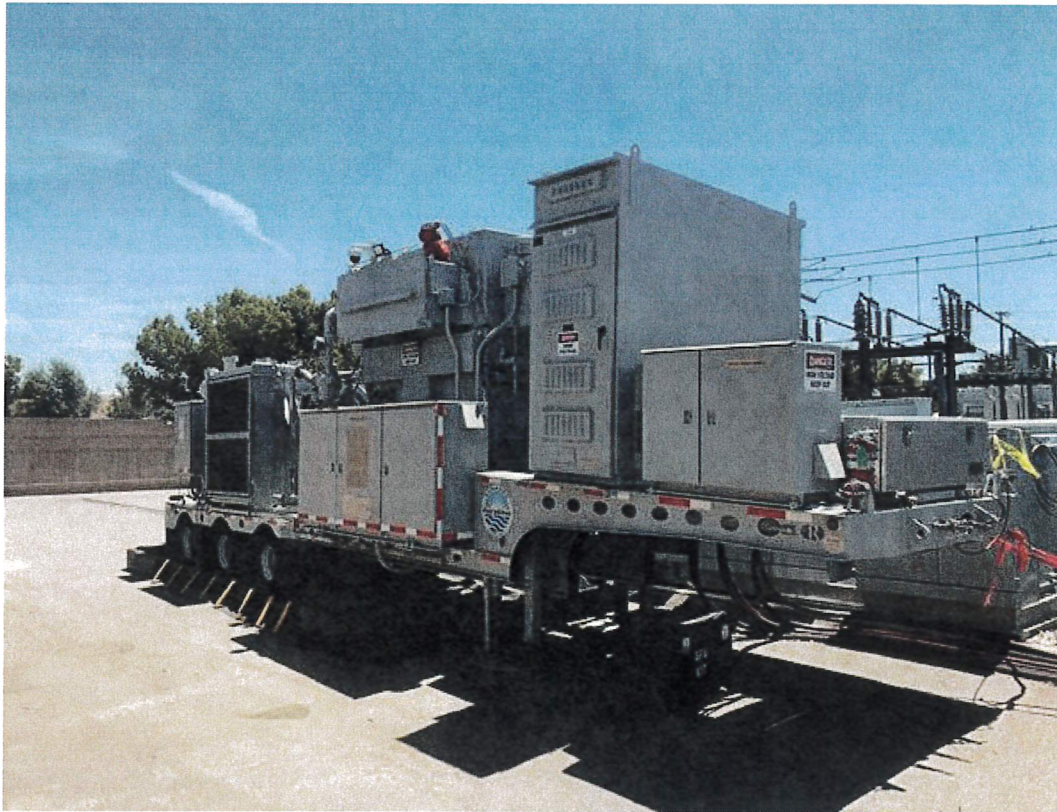
Mobile Substation at Golden State Substation
