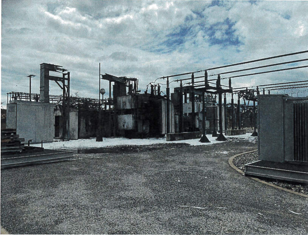
Golden State Substation After Transformer Fire on 4/10/2020
