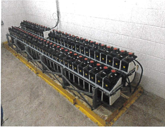
Battery Bank – Before Installation
