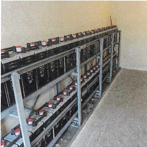
Battery Bank – Before Installation
