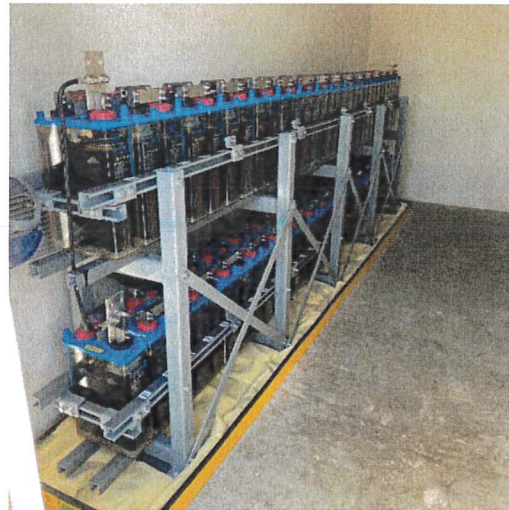
Battery Bank – After Installation
