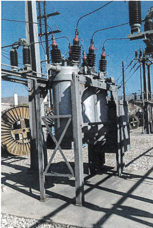
Original 34.5 kV Oil Circuit Breaker at Valley
