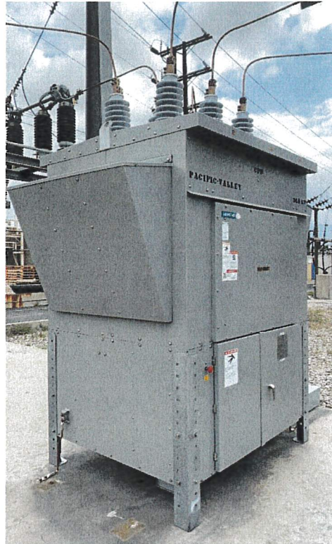
New 34.5 kV Vacuum Circuit Breaker at Valley
