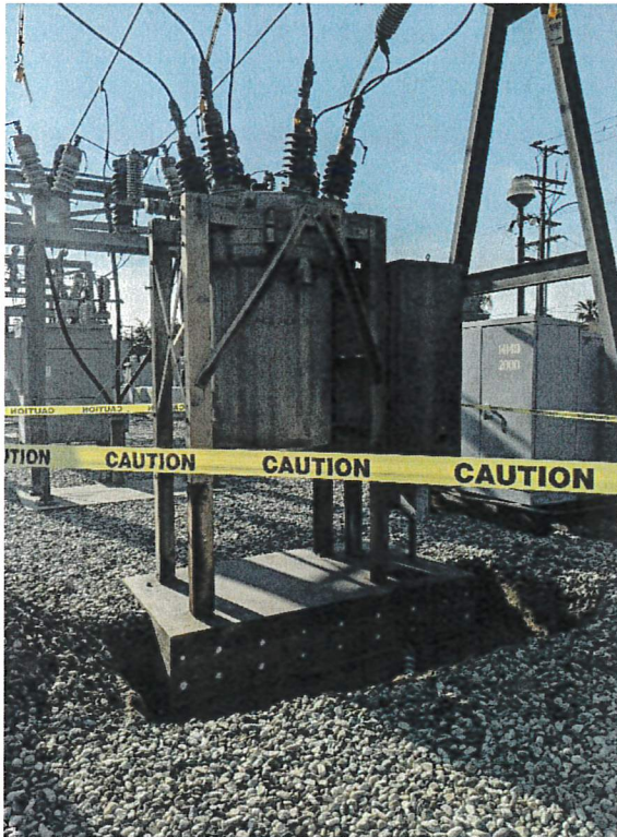
Original 34.5 kV Oil Circuit Breaker at Lincoln
