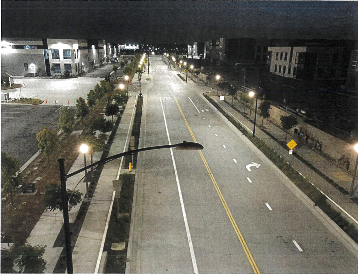
Figure 4 – New street lighting system along Tulare Ave (looking west from Hollywood Way)
