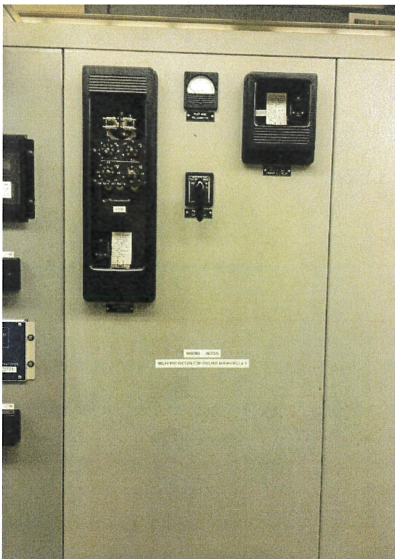
Prior to Replacement (old relays)
