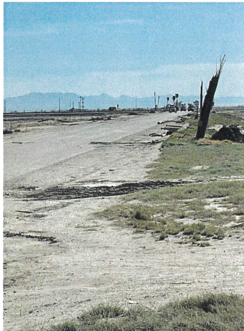
Figure 2 – Broken poles as pictured at arrival to work area
