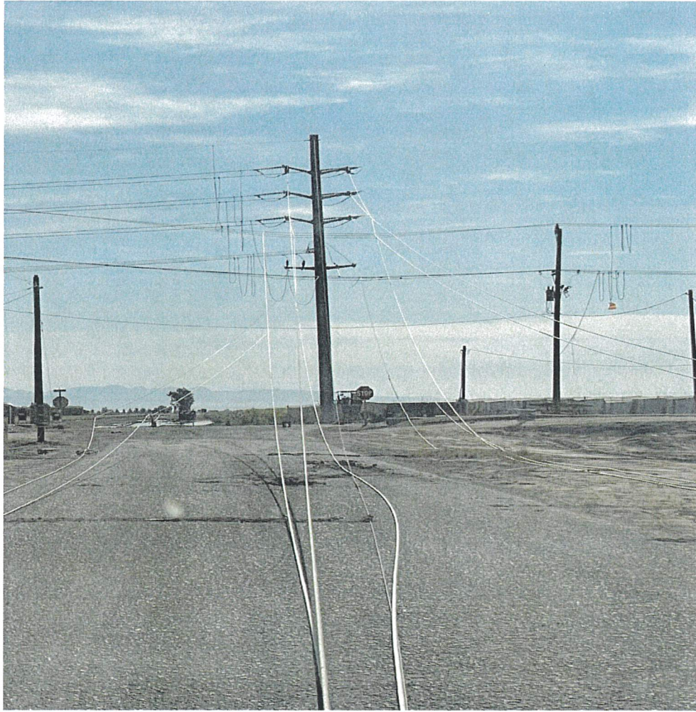
Figure 1 – Fallen wires as pictured at arrival to work area
