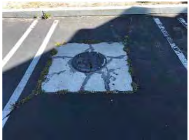
10. View of the groundwater monitoring well on the northeastern corner of the subject property
