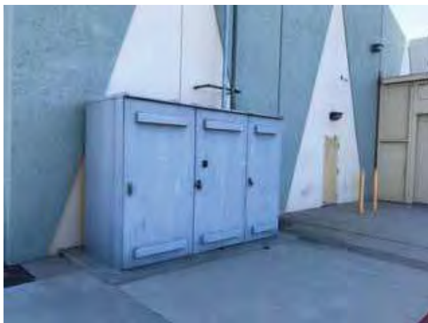
5. View of the subject property electrical panels
