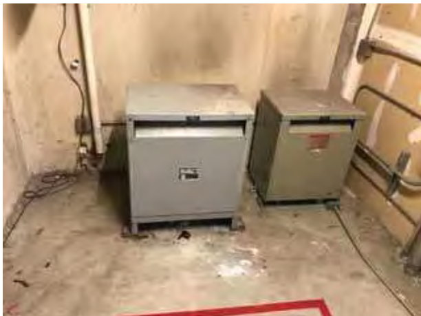
23. View of a typical dry-transformer in the subject property
