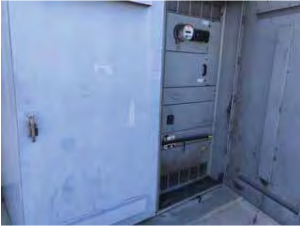
13. View of the internals of the electrical panel
