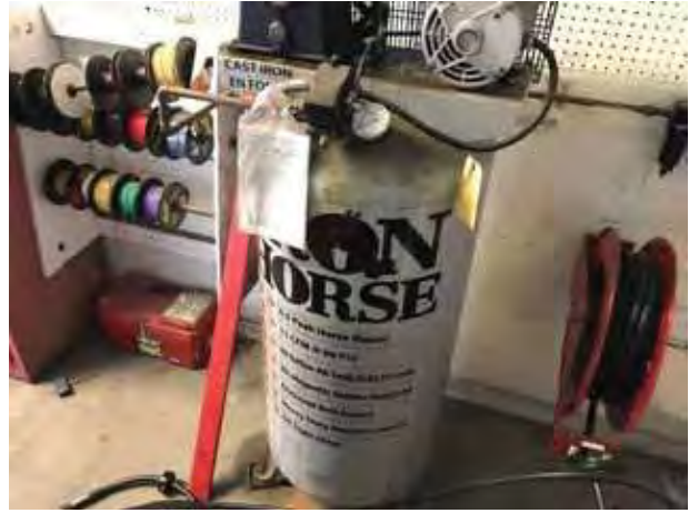
14. View of a not in use air compressor within the automotive stereo installation garage
