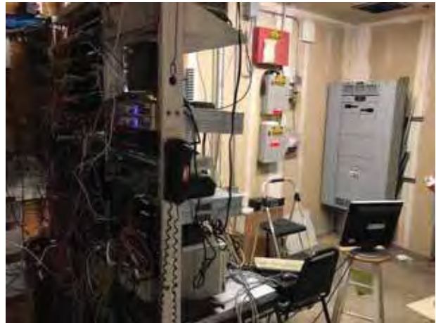
18. View of the central data center and fire sprinkler computer equipment
