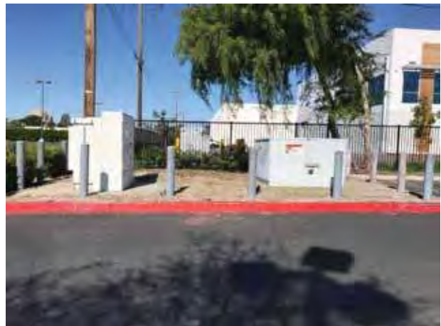
24. View of the two outdoor pad-mounted transformers
