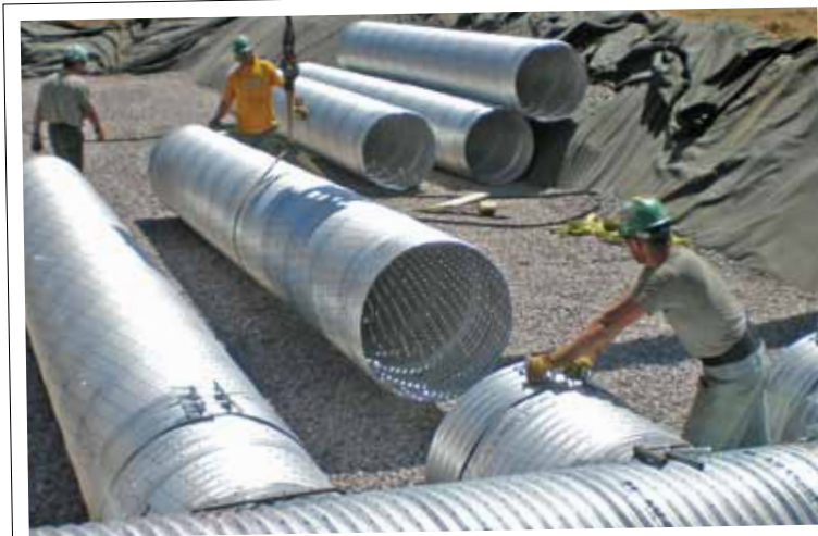
Perforated CMP infiltration system
