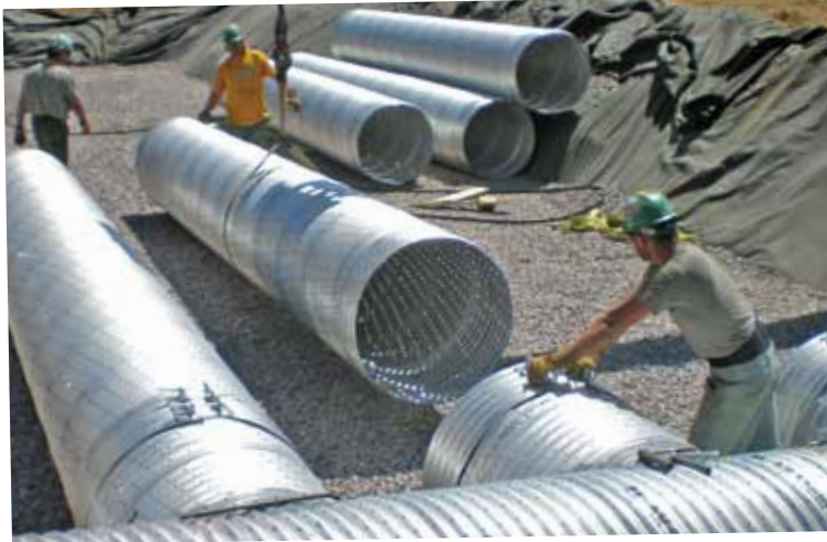
Perforated CMP infiltration system
