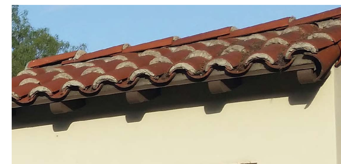
Q. Exposed Decorative Rafter Tails At Bay Window Only w/ 2x3 Wood Fascia
