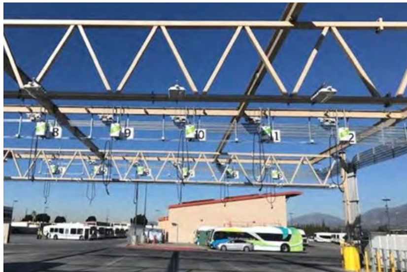
Figure 1-4: Overhead Plug-in Charging Example (Source: Burns McDonnell Foothill Transit In-Depot Charging and Planning Study)
