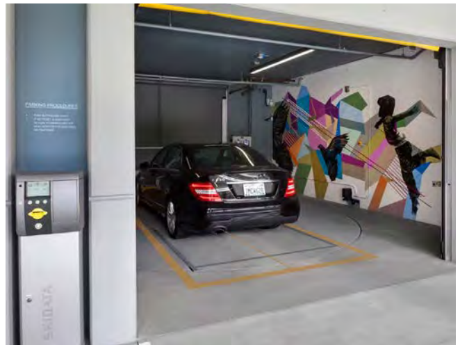
Mechanical parking system
