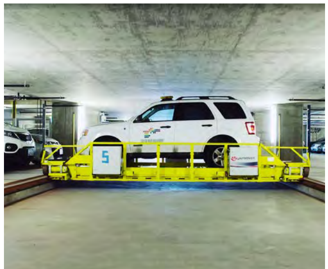
Mechanical parking system
