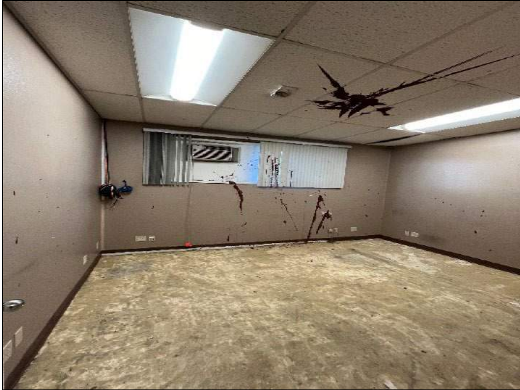
Figure 15: Example of Damage and Vandalism in Primary Structure Interior
